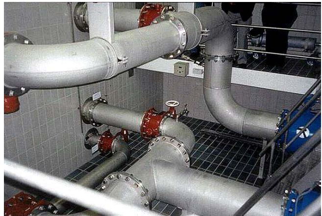
Figure 8. Stainless steel pipework in a water treatment plant. Attention has been given to both good welding and post-fabrication cleaning practices.
