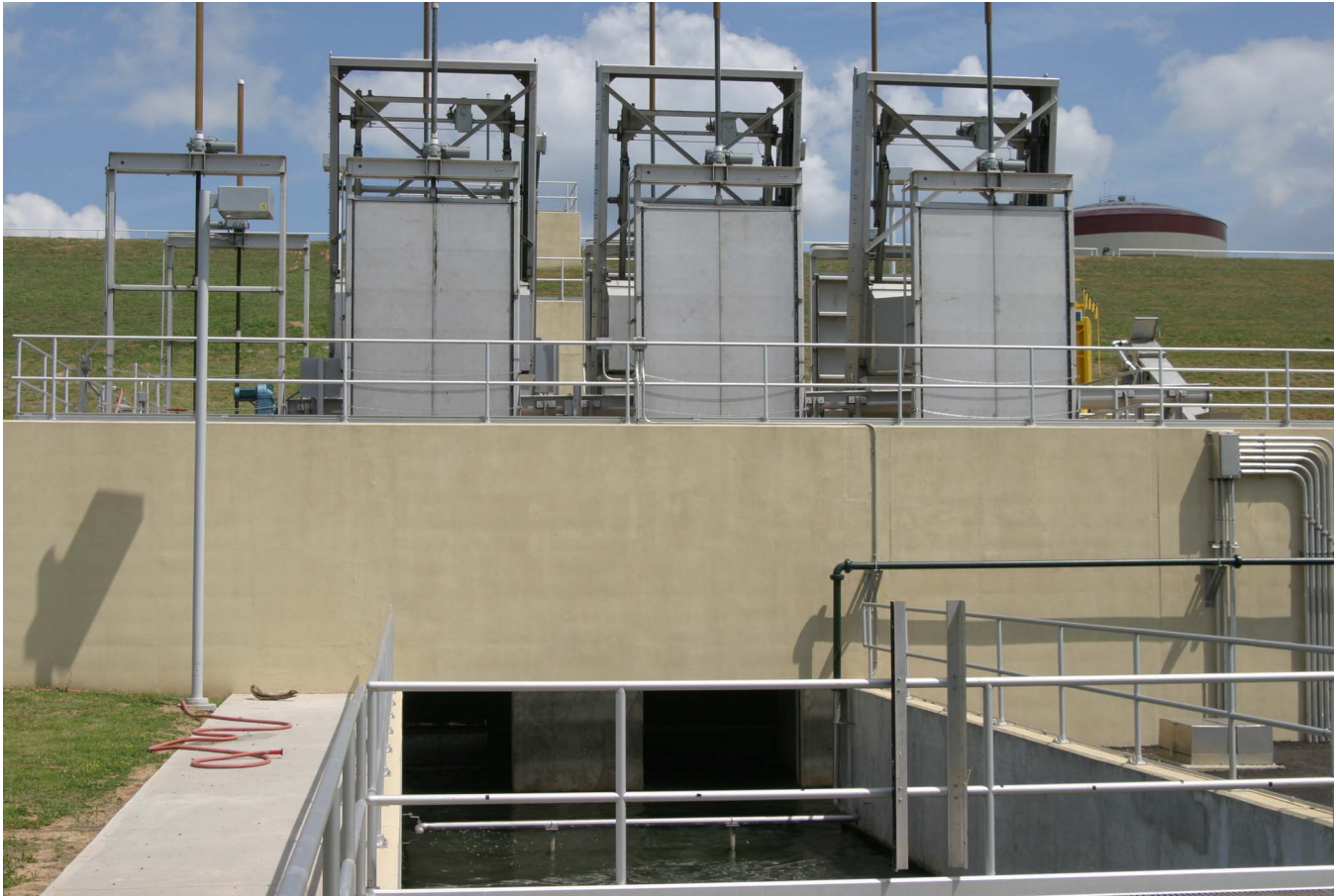
Figure 1. These sluice gates were fabricated of stainless steel and control the flow of waste water between storage basins.
