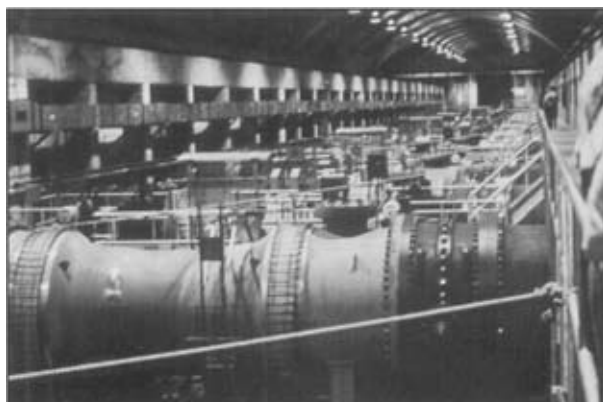
Figure 2 A gallery of laterals in the New York City pumping station. The laterals are made from cast stainless steel with 48 in. diameter wrought butterfly valves.
