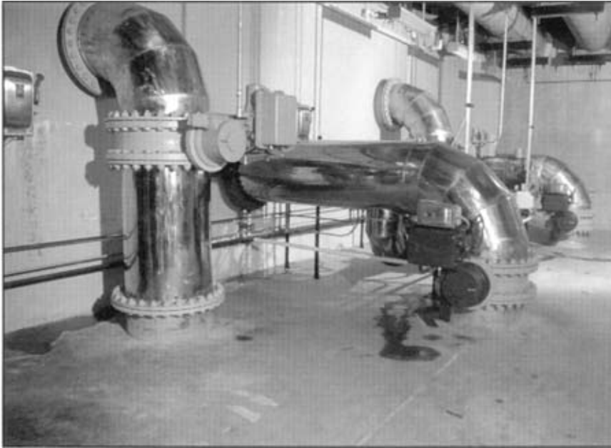
Figure 4 A section of stainless steel piping in the PWTP in Taunton, Massachusetts where cost savings were realized by using lighter weight stainless steel instead of ductile cast iron.
