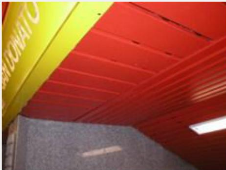
Cladding of the false ceiling in a subway station in Milan, Italy (2006).
